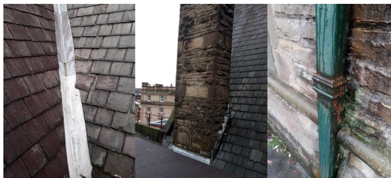
Figure Four – Photos of building defects
